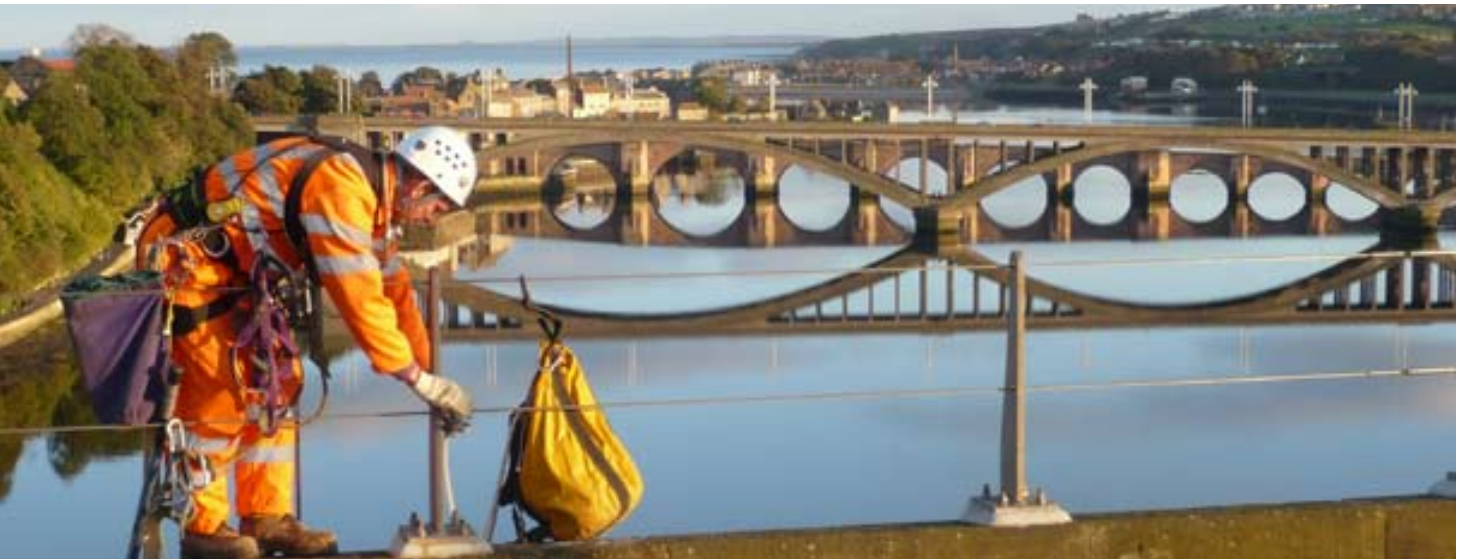
An Amey employee works on the Royal Bridge (Berwick Upon Tweed, United Kingdom)
