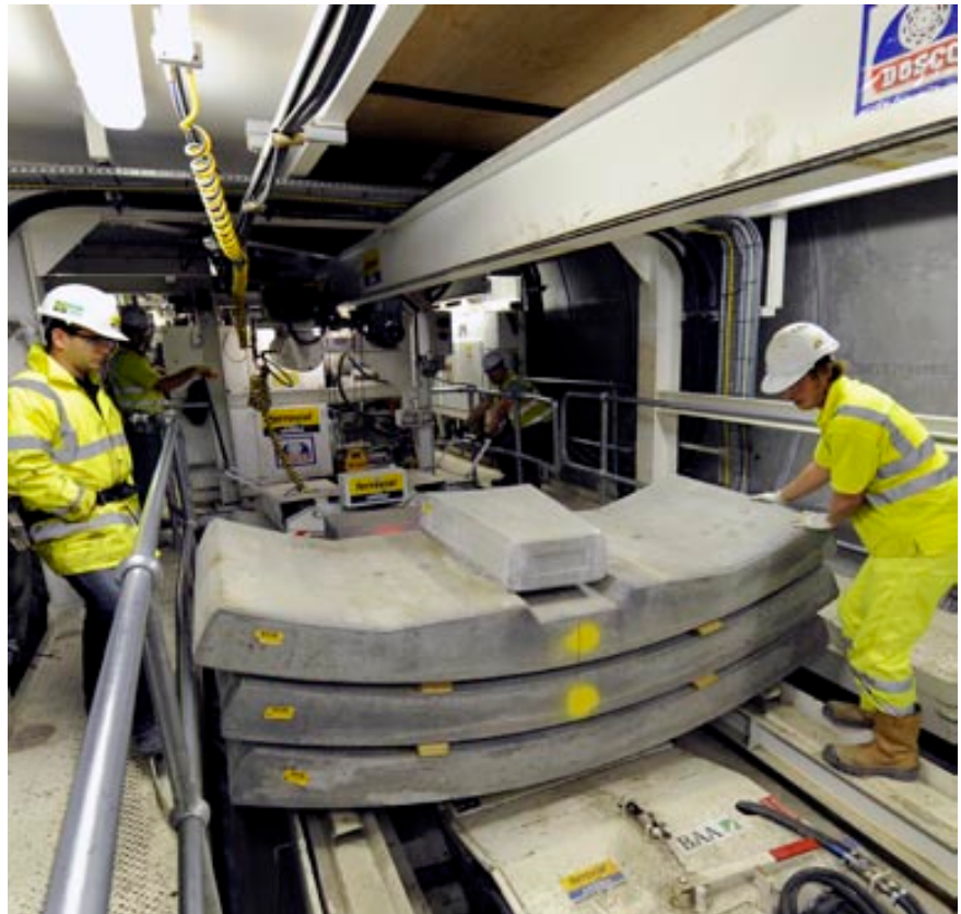
Ferrovial Agromán workers during the construction of a tunnel for the new baggage system at Heathrow airport
