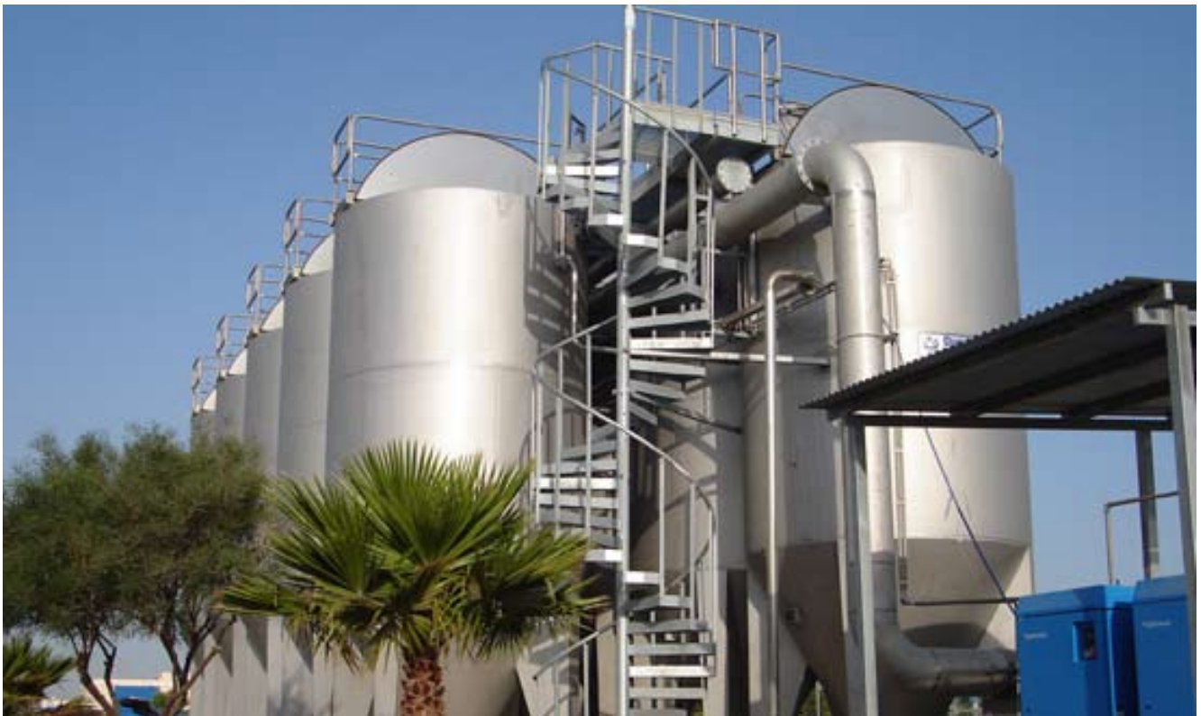
Sand filters of Additional Treatment to EDAR Tertiary Treatment in Campo de Dalias (Almeria, Spain)
