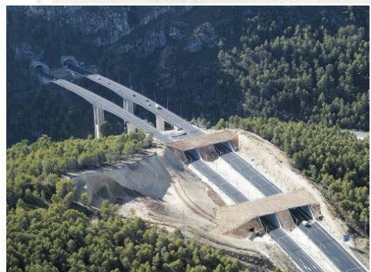
View of the section where the bat crossing protection structure is being installed.
